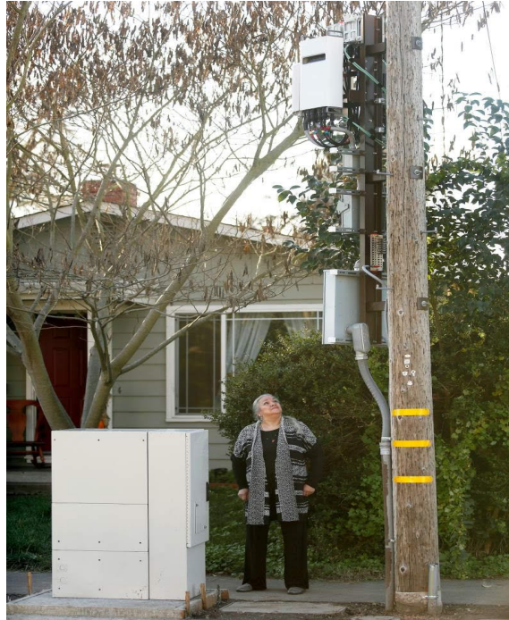
Verizon "Small" Cell installed in Santa Rosa, CA
